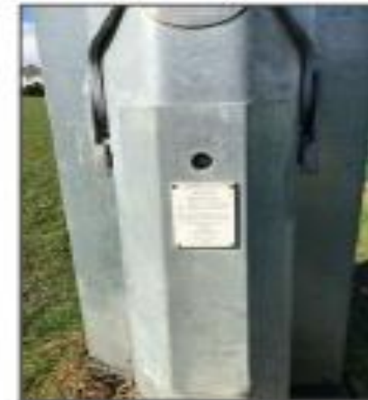
EXISTING ABACUS LIGHTING COLUMNS N.B. EXISTING LIGHTING COLUMNS ORIGINALLY INSTALLED BY HALLIDAY LIGHTING
