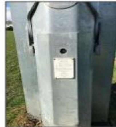
EXISTING ABACUS LIGHTING COLUMNS N.B. EXISTING LIGHTING COLUMNS ORIGINALLY INSTALLED BY HALLIDAY LIGHTING
