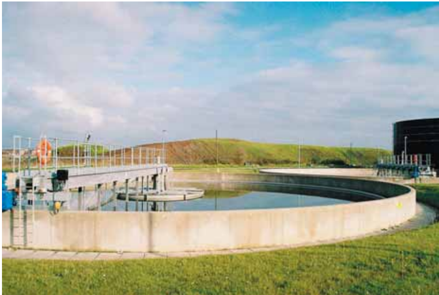
Sewage treatment works, Inchinnan
