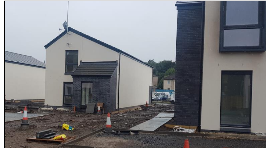
Strategic Housing Investment Plan Project, Link Group, development under construction, Thruscraigs, Paisley
